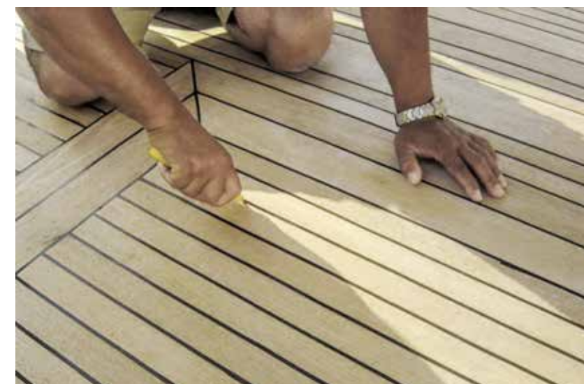
Fig. 60 Using a craft knife to cut along the part of the joint to be removed
